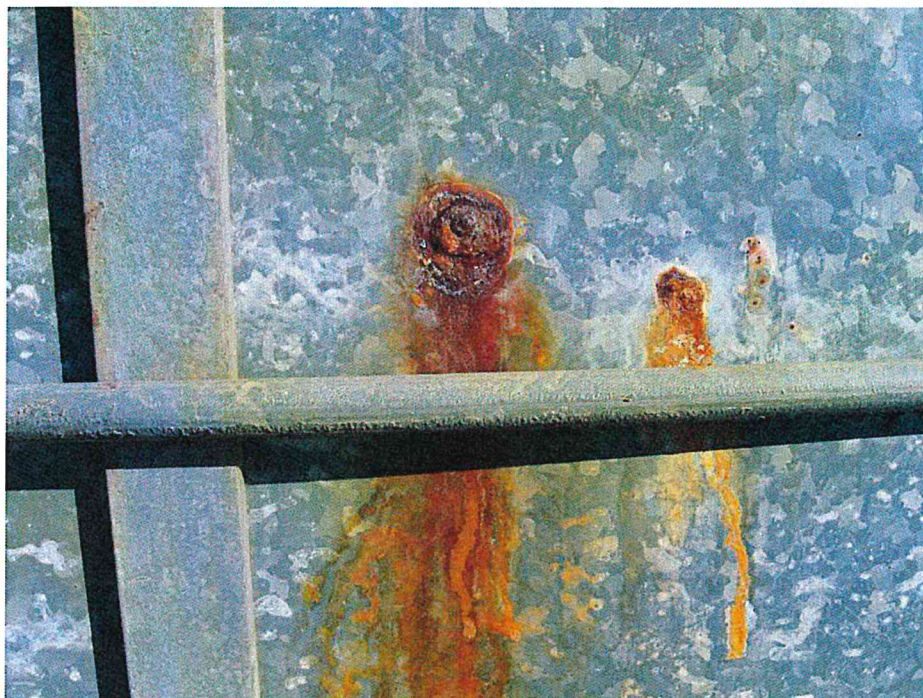
Figure 20 – Spot corrosion West location.
