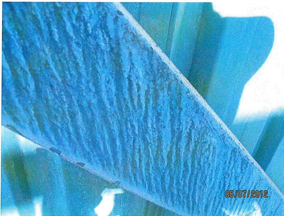
Figure 3 - White residue/scale on steelwork.
