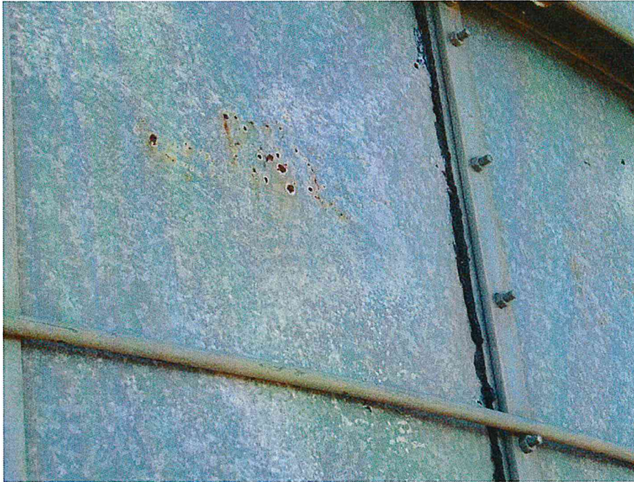
Figure 21 – Typical minor localised corrosion.
