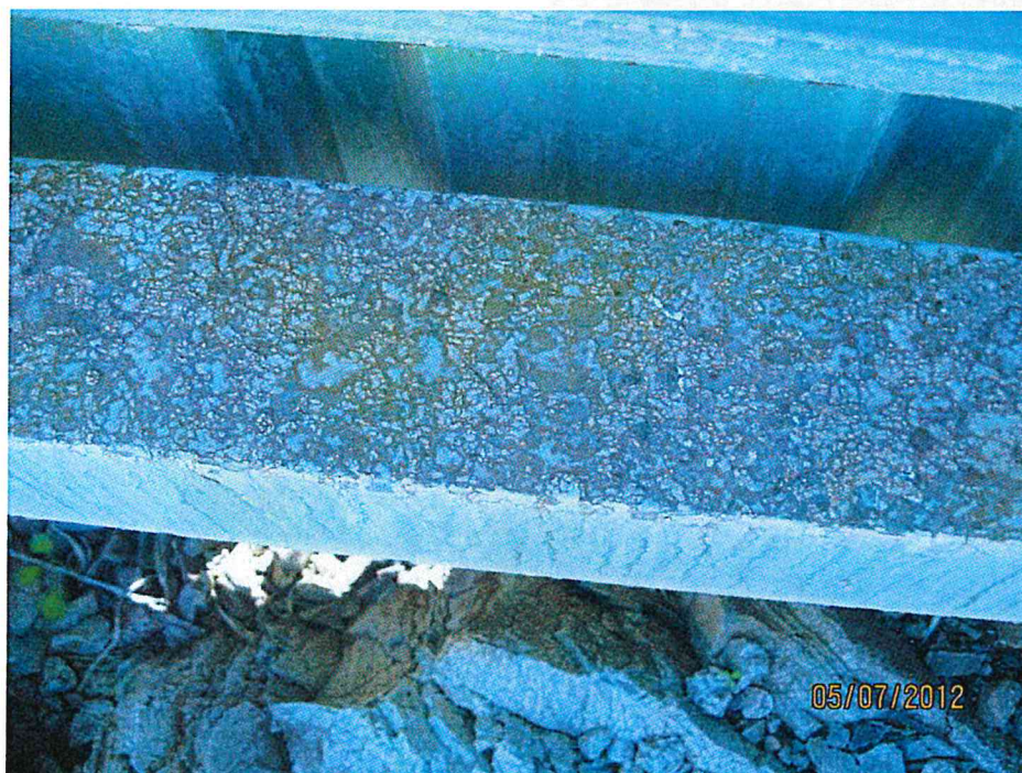
Figure 4 - White residue/scale on steelwork
