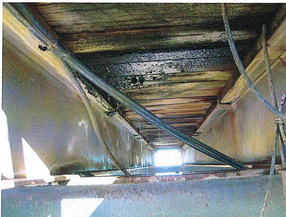
Figure 11 - Timber decking subject to wetting
