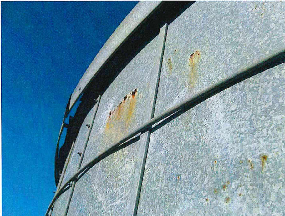
Figure 18 – Full depth shell corrosion North location.
