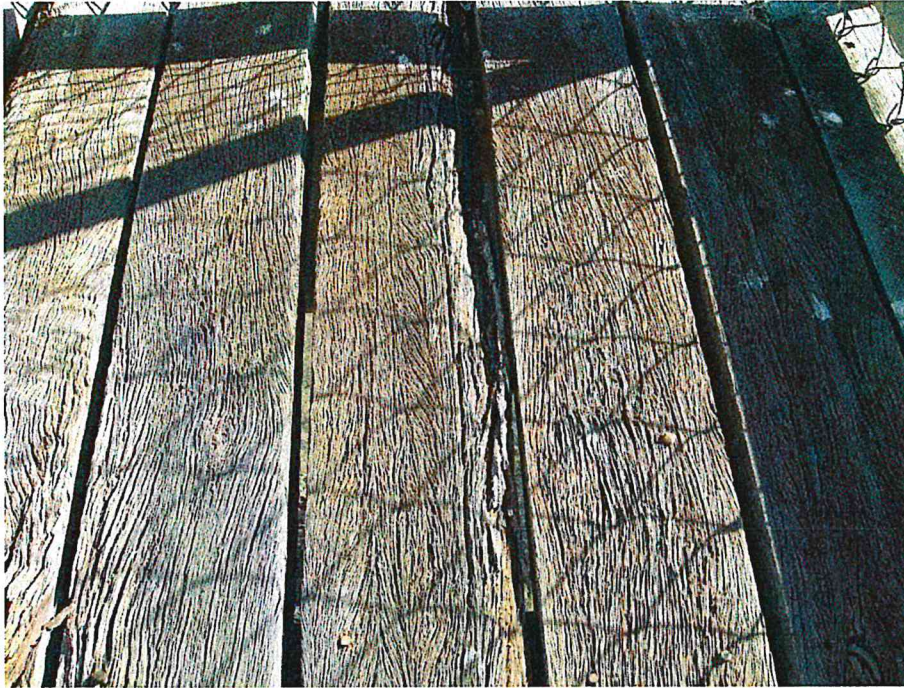
Figure 13 – Timber weathering and splitting
