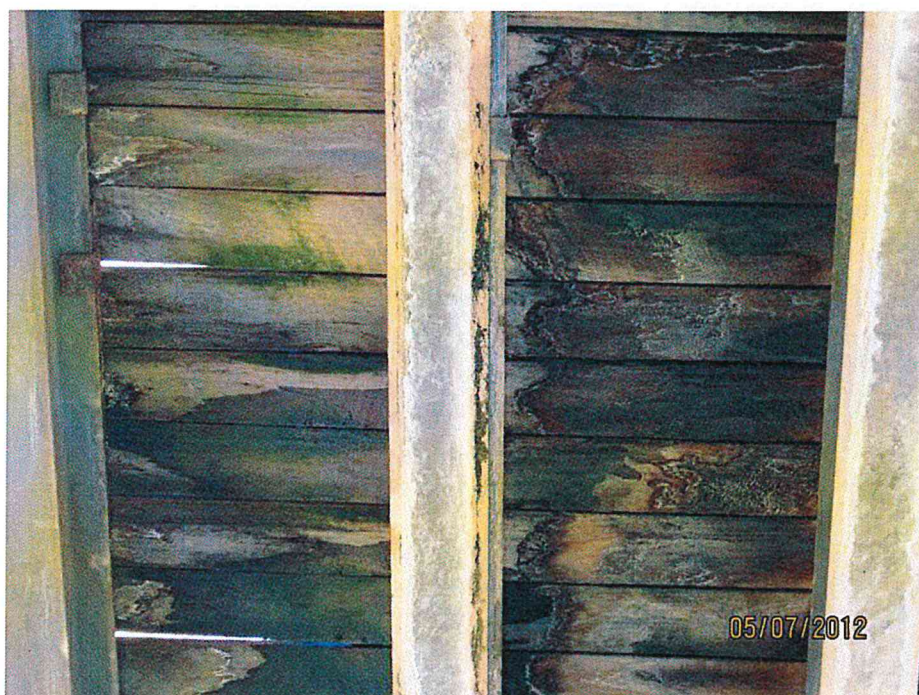
Figure 12 - Timber material defects due to wetting
