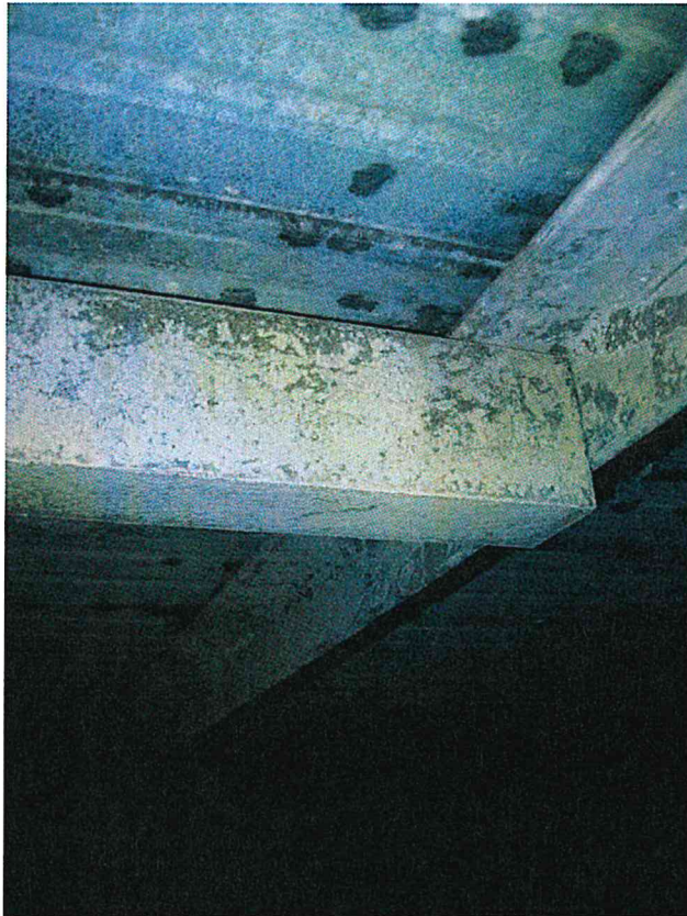
Figure 24 - White residue on internal steelwork and sheeting.
