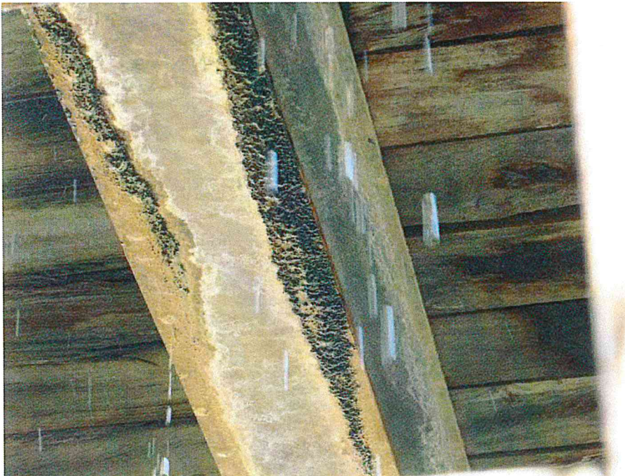
Figure 10 – Black substance on secondary beam.
