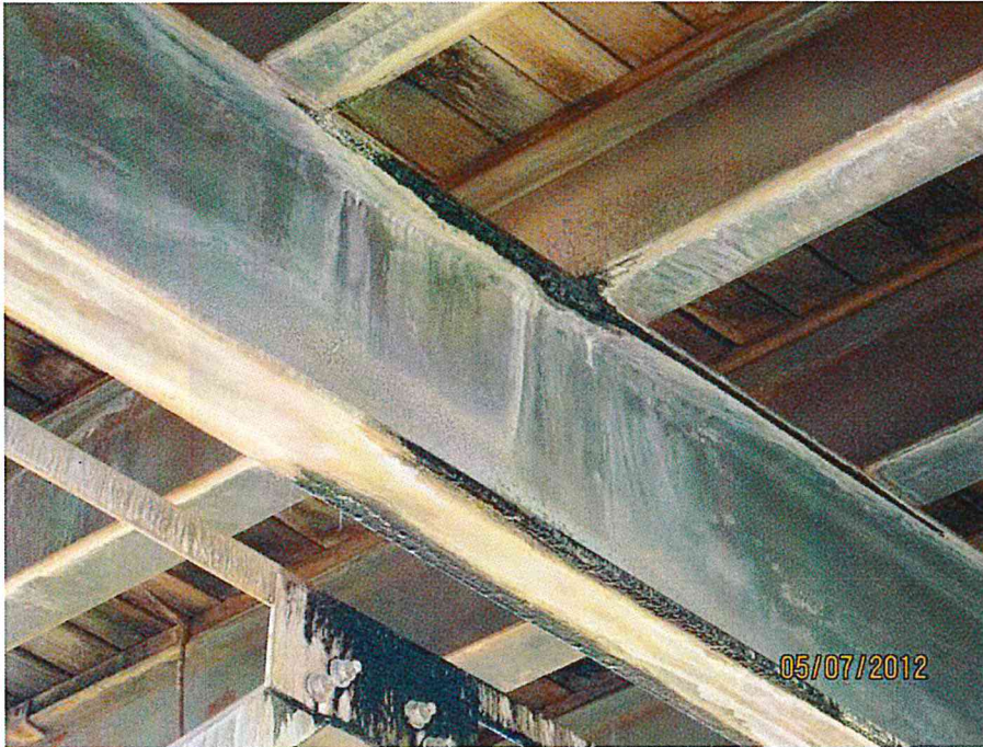
Figure 9 – Black substance on primary beam and adjacent cleat.
