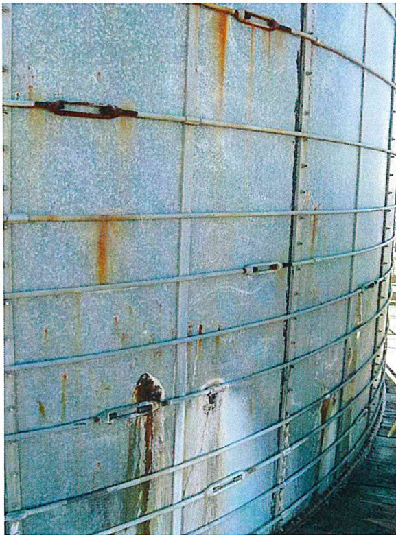
Figure 22 – Turnbuckle corrosion and white residue.
