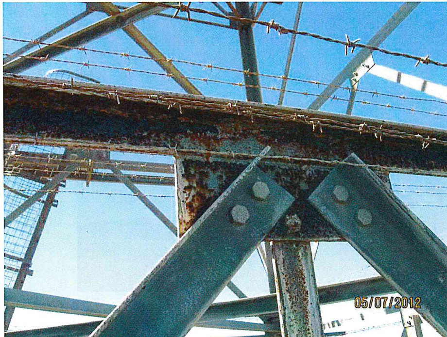
Figure 6 – Corroded angle brace.
