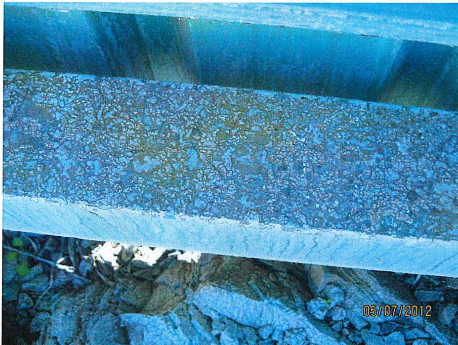
Figure 4 – White residue/scale on steelwork
