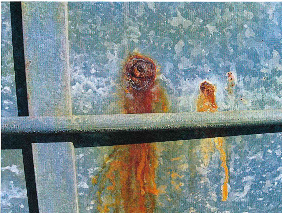
Figure 20 – Spot corrosion West location.
