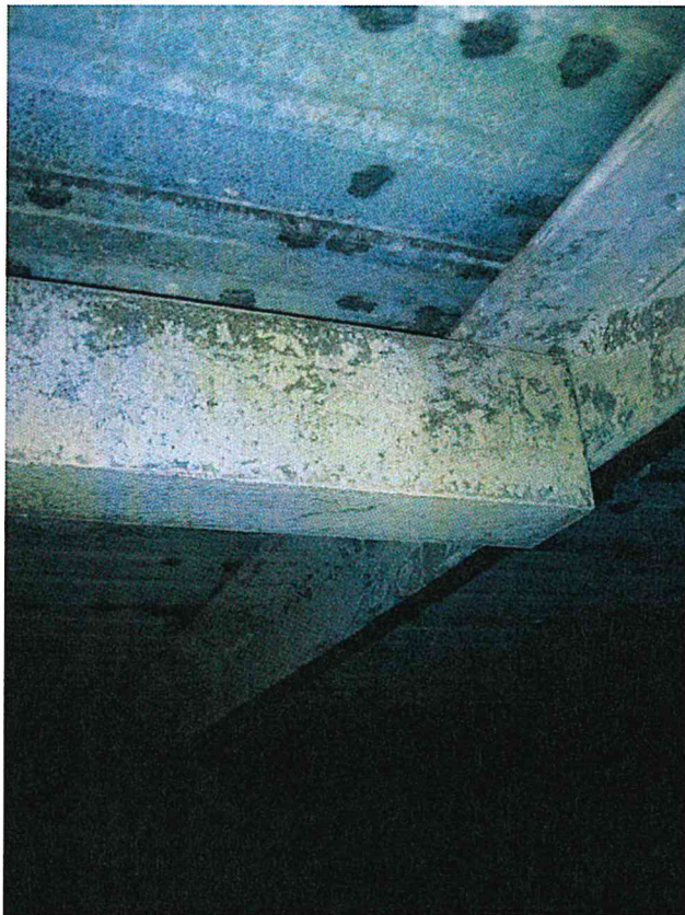
Figure 24 - White residue on internal steelwork and sheeting.
