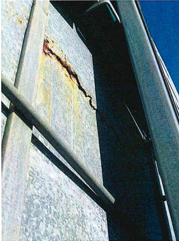
Figure 17 – Full depth shell corrosion North-West location.
