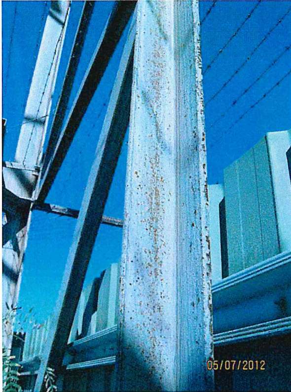
Figure 5 – Minor corrosion typical tower steelwork.
