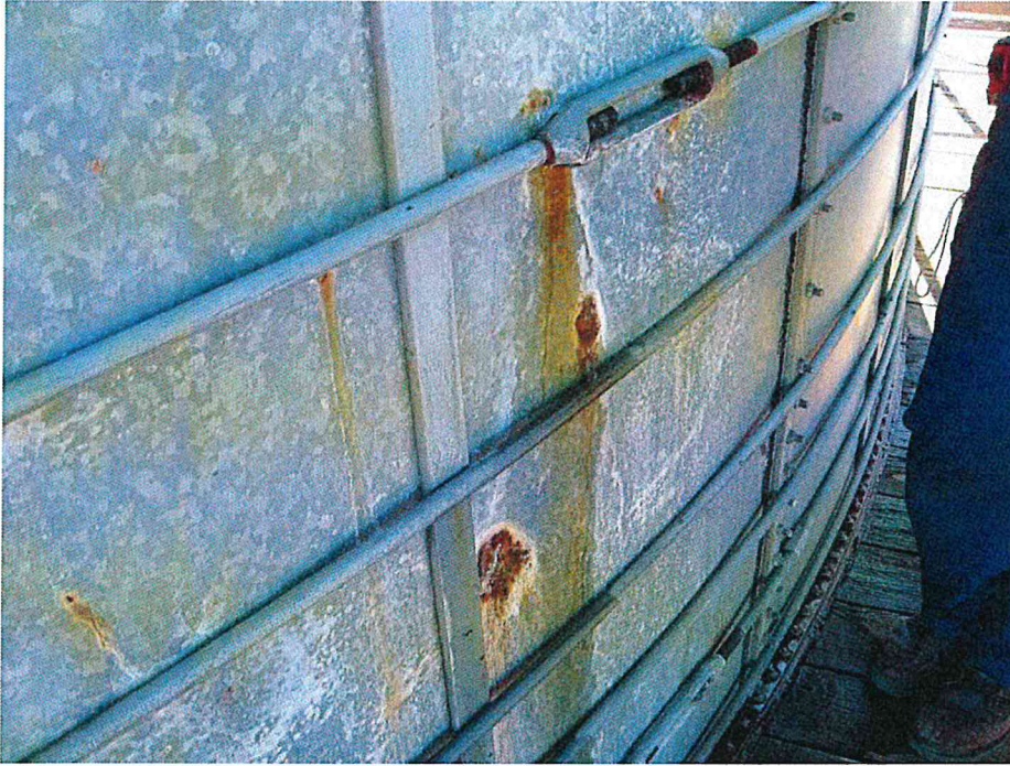
Figure 19 – Typical spot corrosion.
