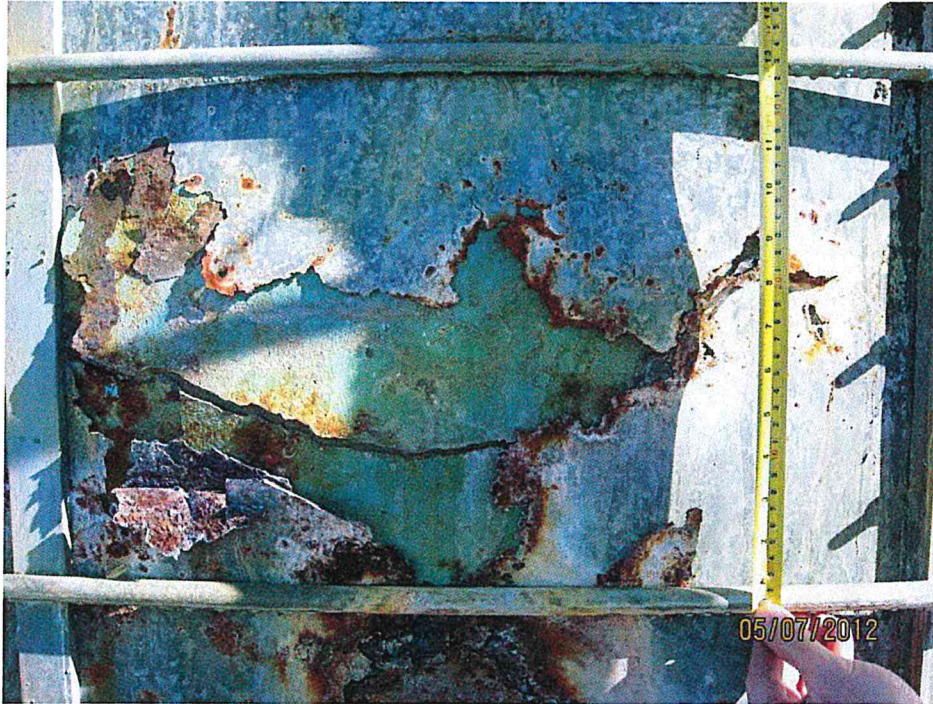
Figure 15 – Full depth shell corrosion North-East location 1 of 2.
