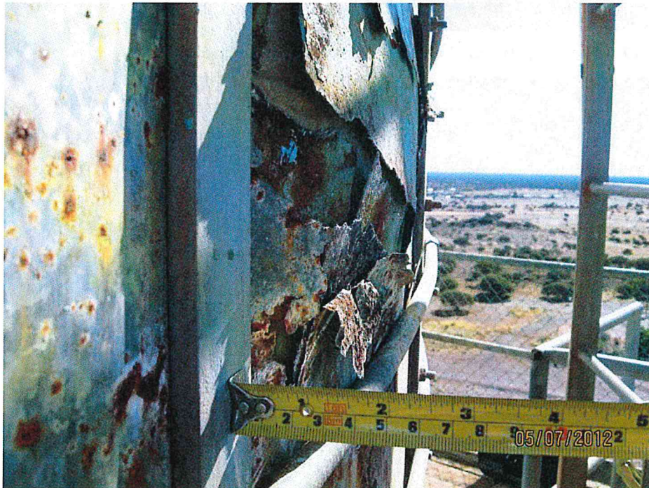
Figure 16 – Full depth shell corrosion North-East location 2 of 2.
