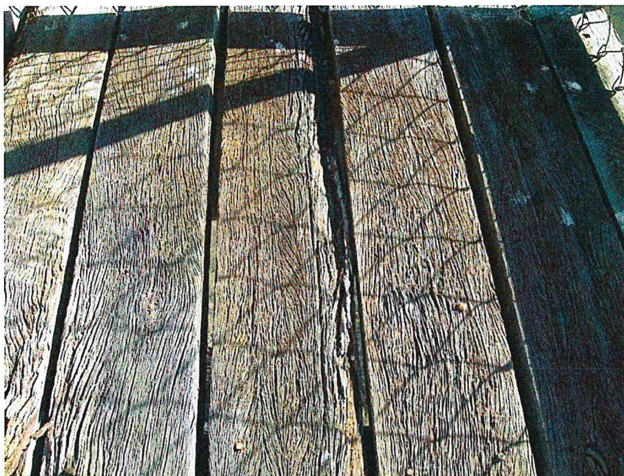
Figure 13 – Timber weathering and splitting
