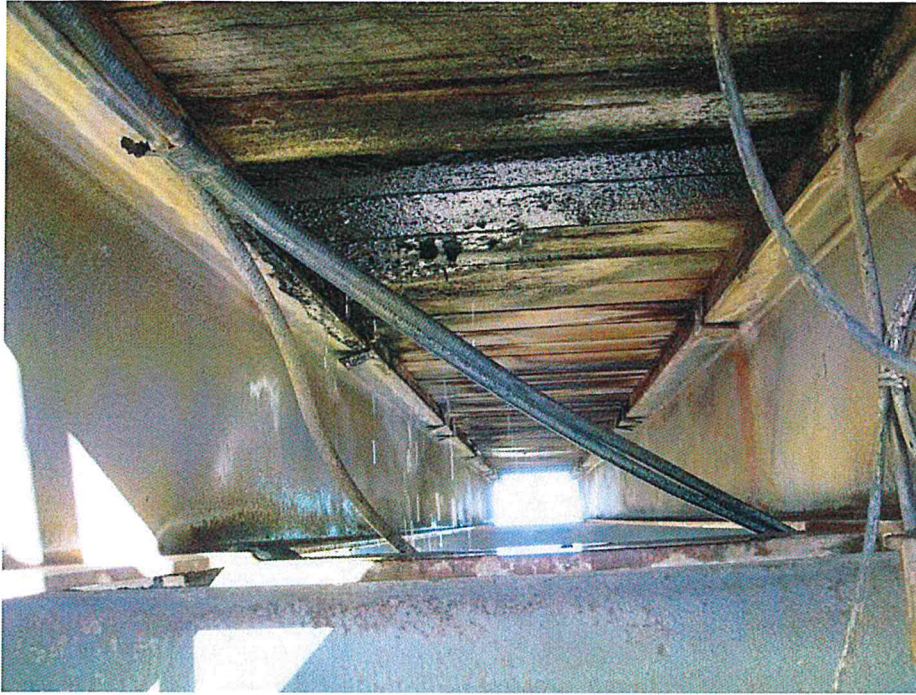
Figure 11 - Timber decking subject to wetting
