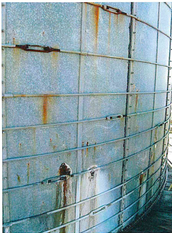
Figure 22 – Turnbuckle corrosion and white residue.
