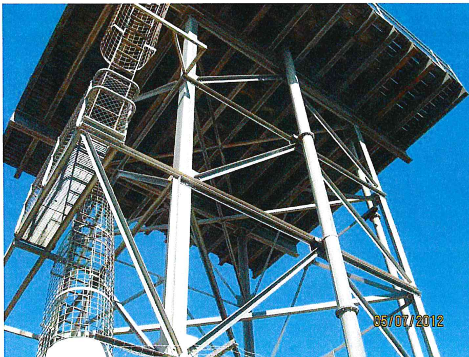
Figure 2 - Platform access system.
